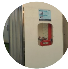
Outdoor emergency washing facility
