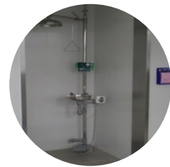
Indoor emergency washing facility
