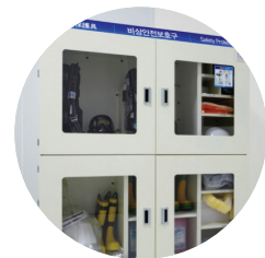
Protective equipment for emergency
